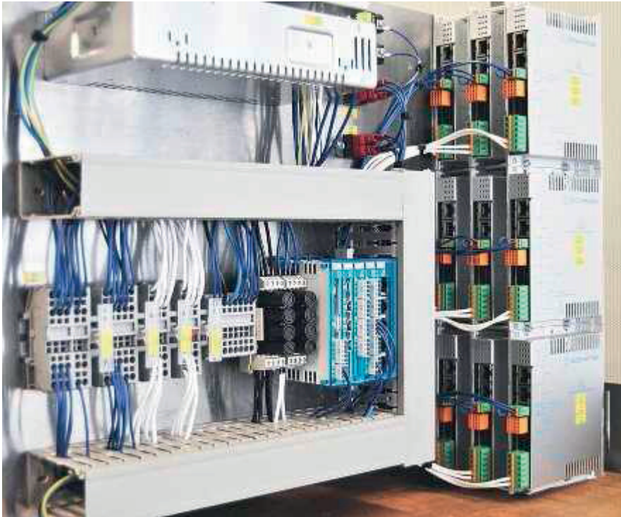
With the 3D printer 140L, the entire automation system is contained in a single control box. On the right, up to twelve axes are mounted.
