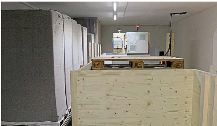
Automated warehouse management with isofloc industrial bales. In the background, the control cabinet for the blow-in module.
