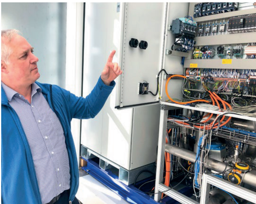
Bernd Maus at the control cabinet. He emphasizes: 'The excellent, direct support was an important factor in our decision to work with SIGMATEK.'
